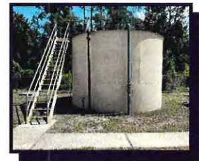
Sludge Holding Tank
