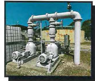
Transfer Pump Station
