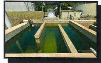
Chlorine Contact Chamber
