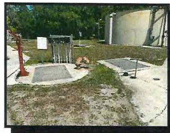
Master Lift Station
