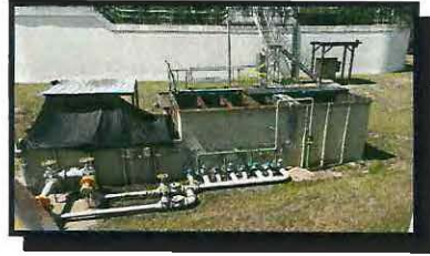
Tertiary Filtration System
