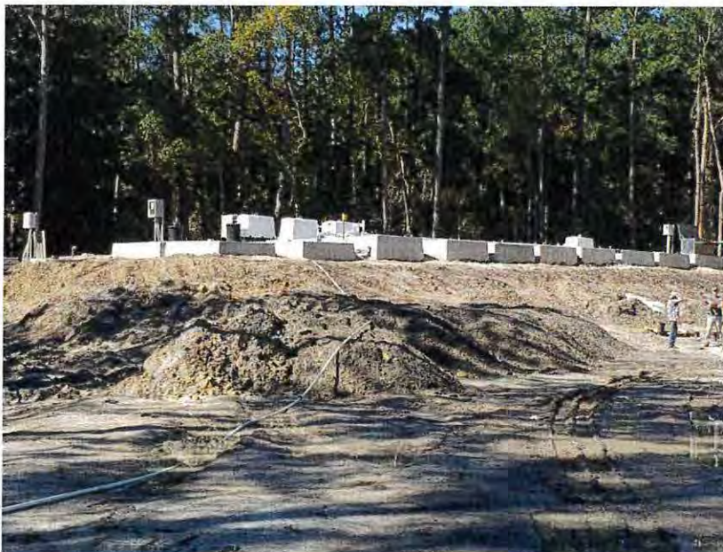
Island Oak Wastewater Treatment Plant
