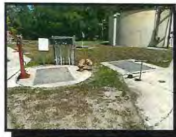
Master Lift Station
