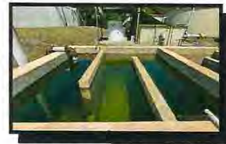
Chlorine Contact Chamber
