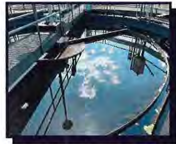
Secondary Clarifier (BTU)
