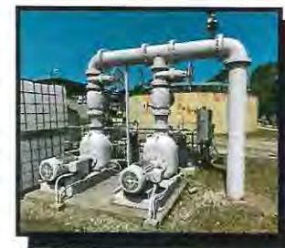
Transfer Pump Station
