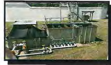
Tertiary Filtration System
