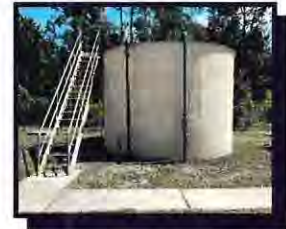
Sludge Holding Tank
