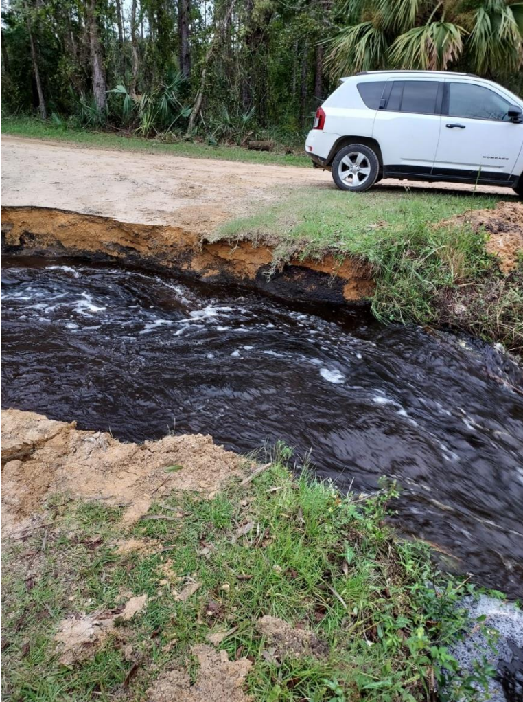
450 Old Haw Creek – Driveway washout after Ian
