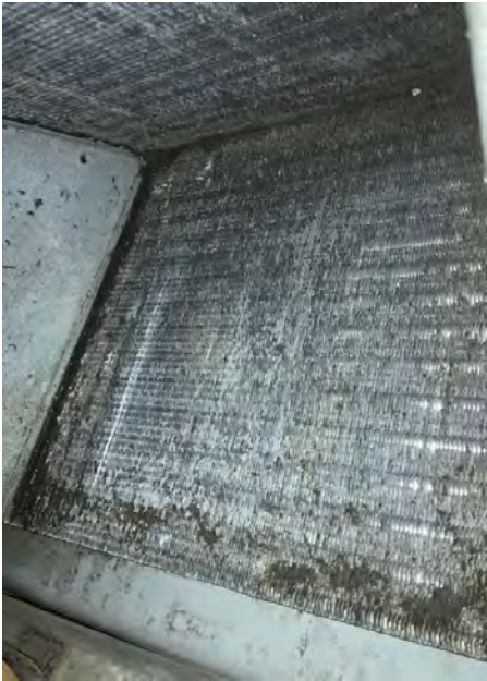
Unit #2 evaporator coil
