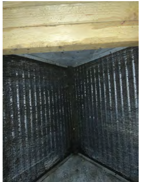
Unit #2 evaporator coil
