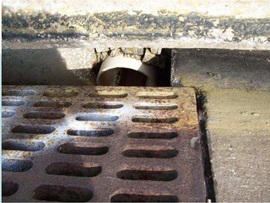
Unknown Pipe Into Storm Sewer Inlet
